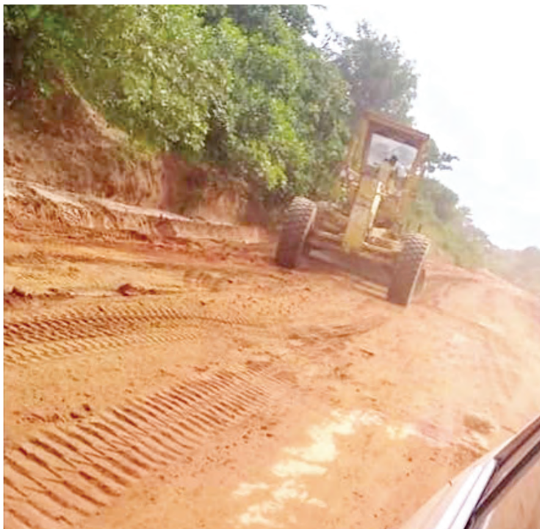
■ A heavy duty grader being used to rehabilitate the Enjema to Okobo road by Zuma 828 Coal Ltd recently
