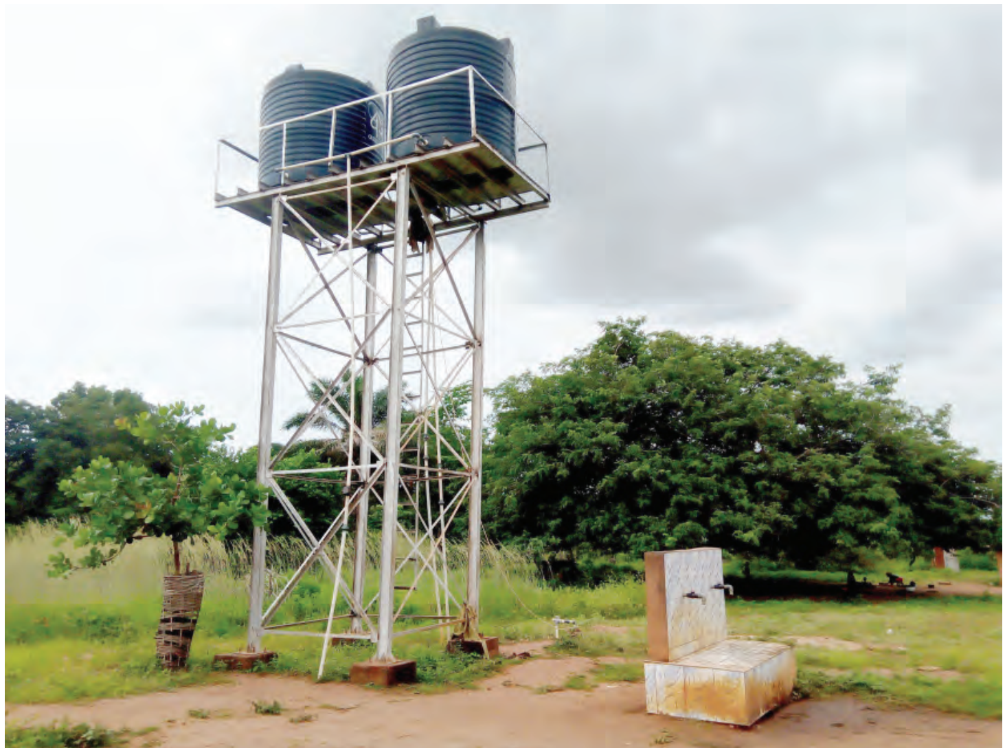
■ Functional borehole donated by Zuma 828 at Okobo Ate community near Okpiko mine site
