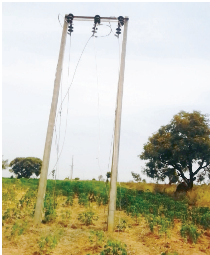
■ Vandalised cables which were to link Mutum Biyu with the National Grid from Jalingo, the state capital
