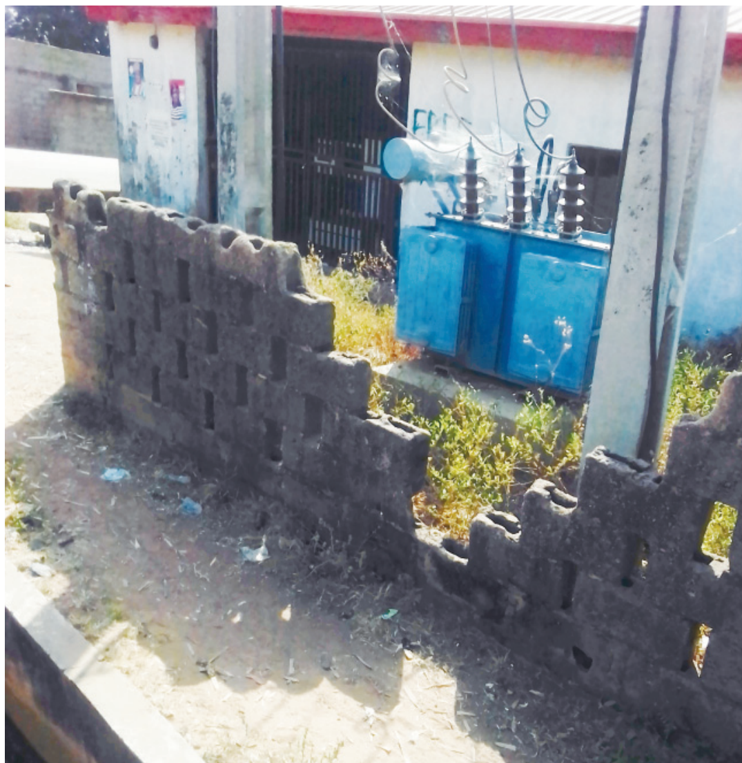
■ The engine room that supplies electricity to Mutum Biyu town, headquarters of Gassol Local Government Area of Taraba State
