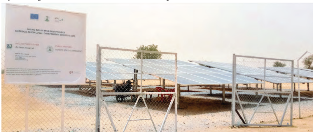
■ The solar power plant at Kurdula community in Sokoto State
