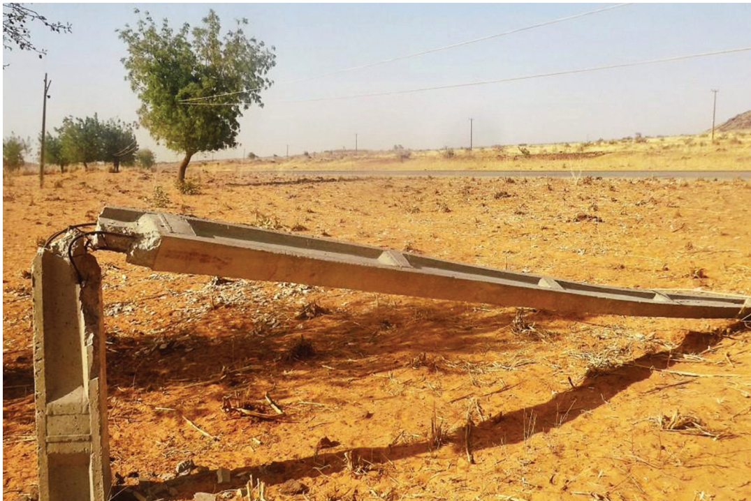
■ An electric pole that fell along Gidan Madi-Silame road
