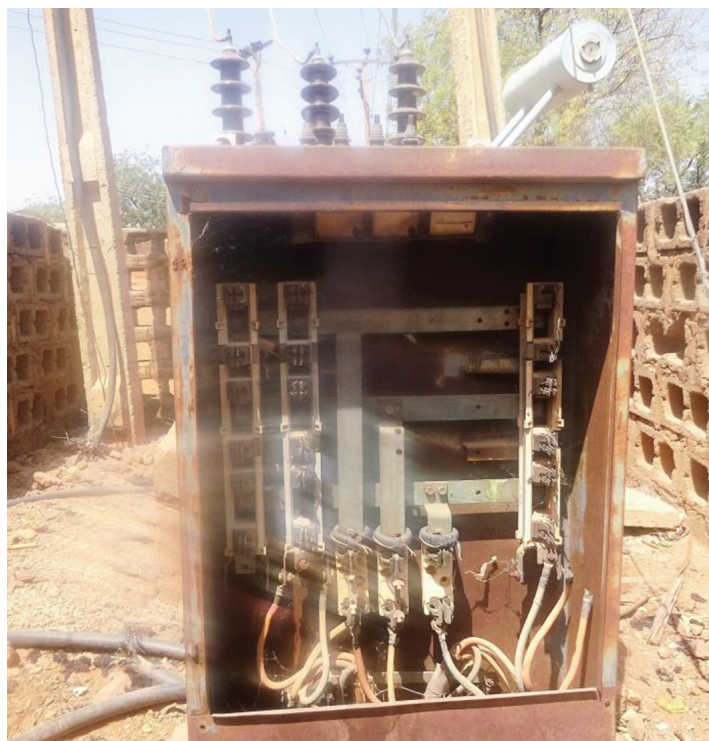
■ A vandalised transformer at Silame
