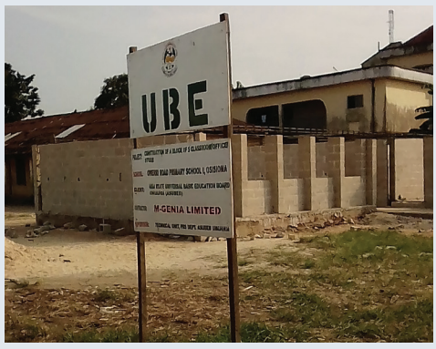
Fig 1.4: Construction of a block of 5 classroom Owerri Road Primary School 1 Osisioma By UBE
