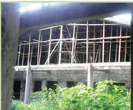
Fig 3.10. Referral General Hospital Ogbia Town still under construction for years after award
