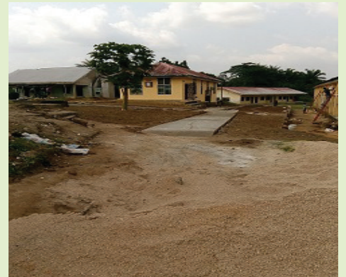
Fig 2.6: An erosion control work and remedial work carried out by the authorities of the School of Health Technology, Etinan
