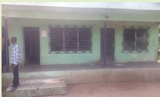
Fig 2.7 The rented apartment used as the Government Vet Clinic at Ikot Akpan Nkuk
