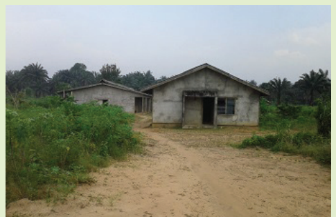
Fig 2.9. The two existing pig pens at the pig farm, Ikot Ibritam, Oruk Anam
