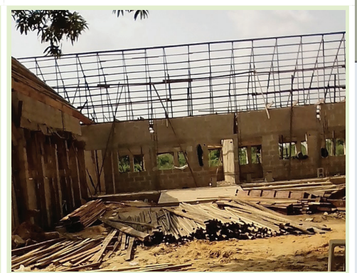
Fig 1.3: Construction of classroom blocks, Abayi Umuocham Boyes High School, Osisioma by ASUBEB
