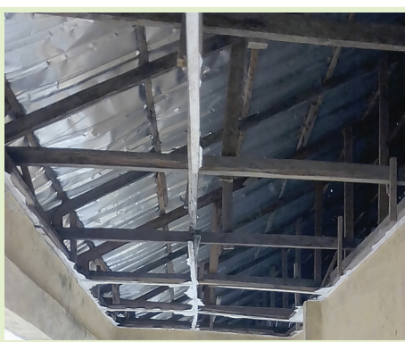
Fig 1.1: dilapidated roof of Ogor Hill primary school iii, Ogor Hill Aba.
